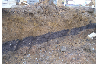
Fig. 13. A weathered coal seam (about 20 cm thick) in the excavation for the foundations of the building. It is clearly part of a separate basin, now almost 100 meters above the main basin. The Kohlbruch connection cannot be proven
