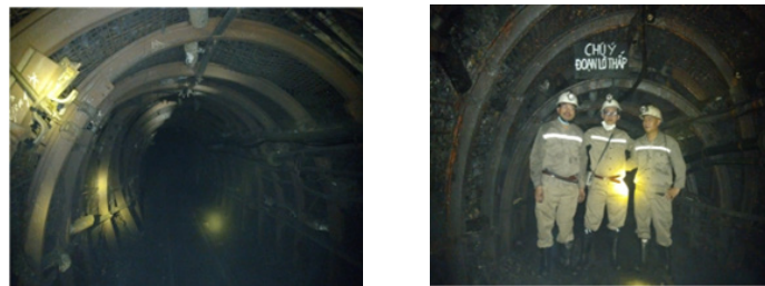
Fig. 6. Some typical failures in DVTG 14.4-2 tunnel at Khe Cham III coal mine in 12/05/2021 in Quang Ninh coal mine area at [1] (by authors)
